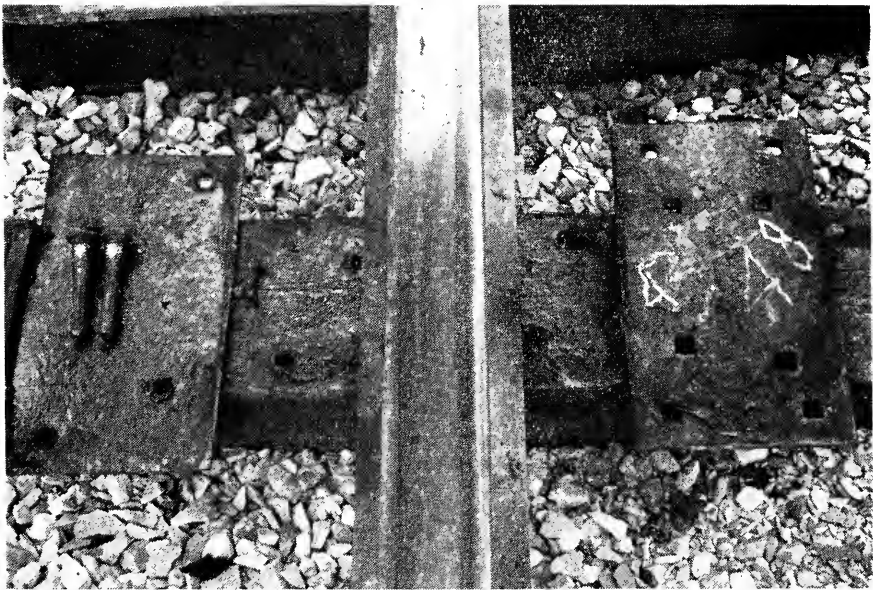
Fig. 21. Section 48. 14-in Racor Tie Pad, Coated, and Racor Studs, After 23-months' Service in the Inner Rail of the Long 4-1/2° Curve
